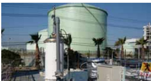
Hydrogen sulfide removal
